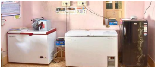
Health centres piloting DRE cold chain solutions
